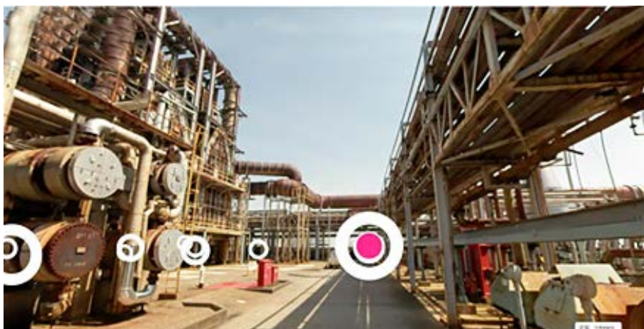
Fig. 1: An oil refinery plant captured as a digital twin. Cosmo Oil (Japan) consolidated three refineries into one virtual model, enabling remote collaboration and “increased efficiencies... and maximized productivity” across its engineering teams. (Source: Cognite.com)
